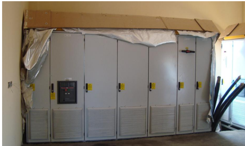
Figure-2: Solar Inverters (ABB make) erected in CMCS Building of P-2 Block as on 29.02.2016
