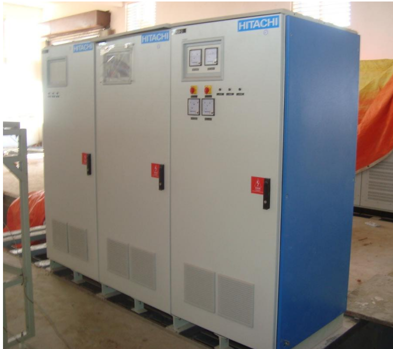
Figure-4: UPS (Hitachi make) erected inside CMCS building of P-3 block (M/s Lanco) as on 29.02.2016
