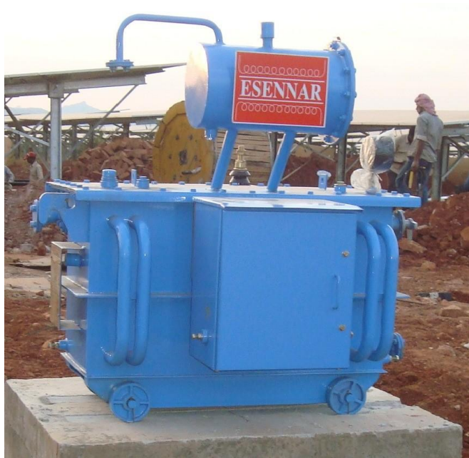
Figure-6: Auxiliary Transformer (esennar Make) erected near CMCS building in P-4 block (M/s BHEL) as on 29.02.2016
