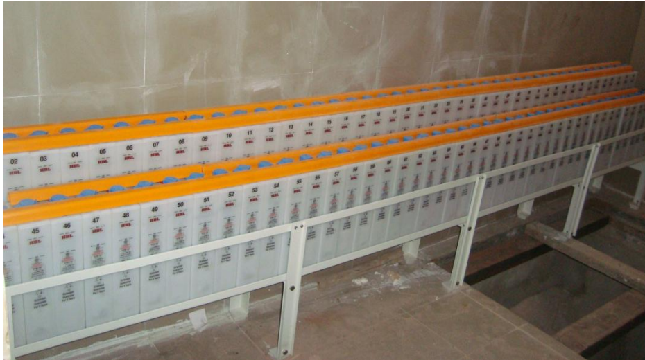
Figure-5: Main battery Bank (110 V, HBL Make) erected in CMCS building of P-3 Block (M/s Lanco) as on 29.02.2016
