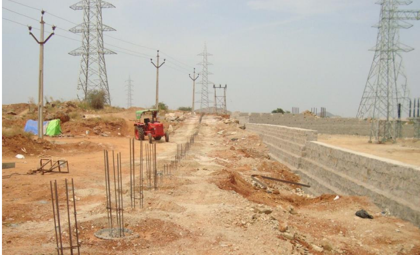
Figure-7: 33 KV Cable Support Pedestals near 220 / 33 KV SubStation of APTRANSCO( M/s APSPCL ) as on 29.02.2016
