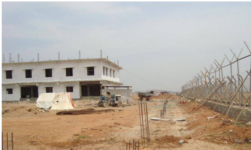
Figure-8: 33 KV Cable Support Pedestals near 220 / 33 KV Sub Station control room of APTRANSCO ( M/s APSPCL) as on 29.02.2016
