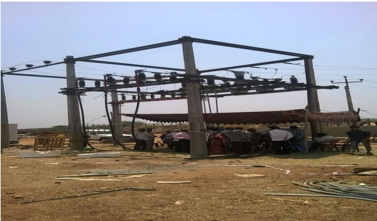
33 kV Sub Pooling Station
