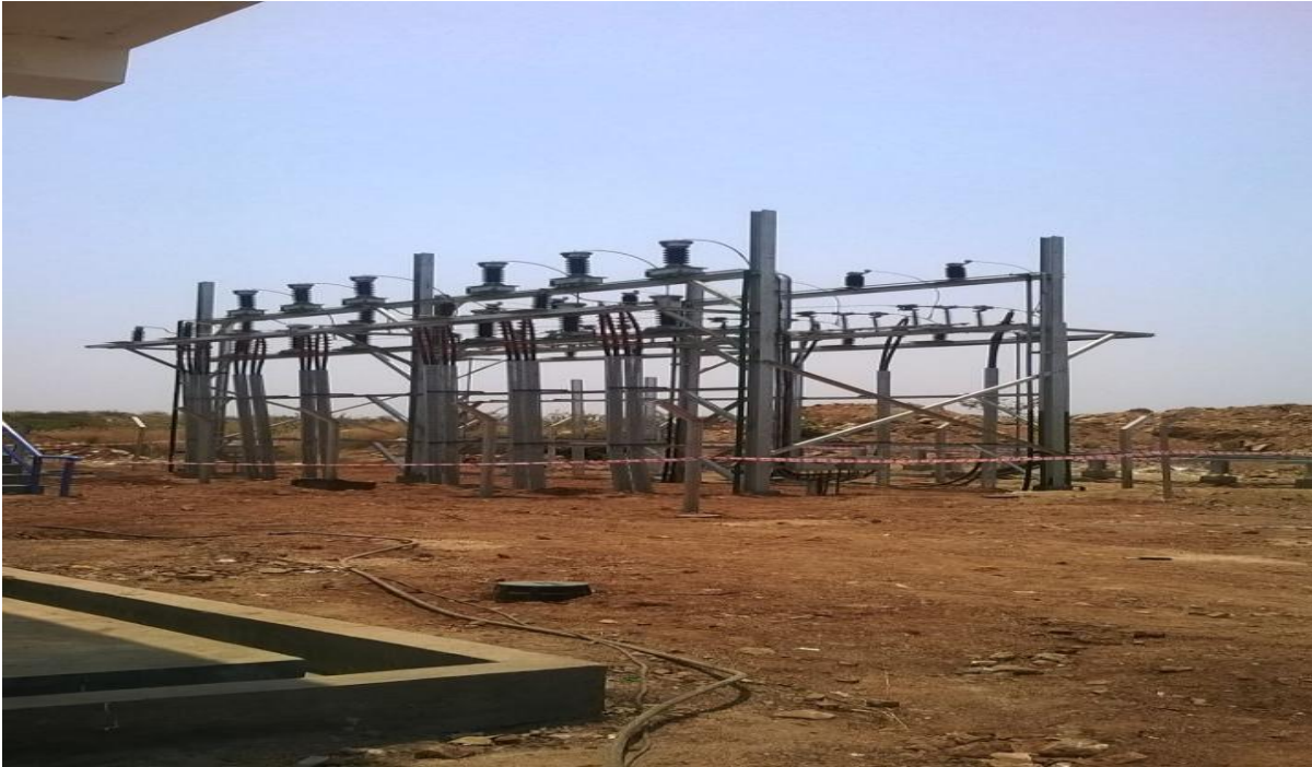
33 kV Sub Pooling Station
